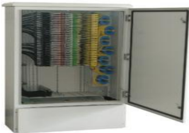
Gambar 3 Optical Distribution Cabinet (ODC) [8]
